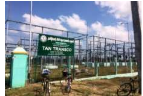
110kV Substation at OneHub Chennai Industrial Park
