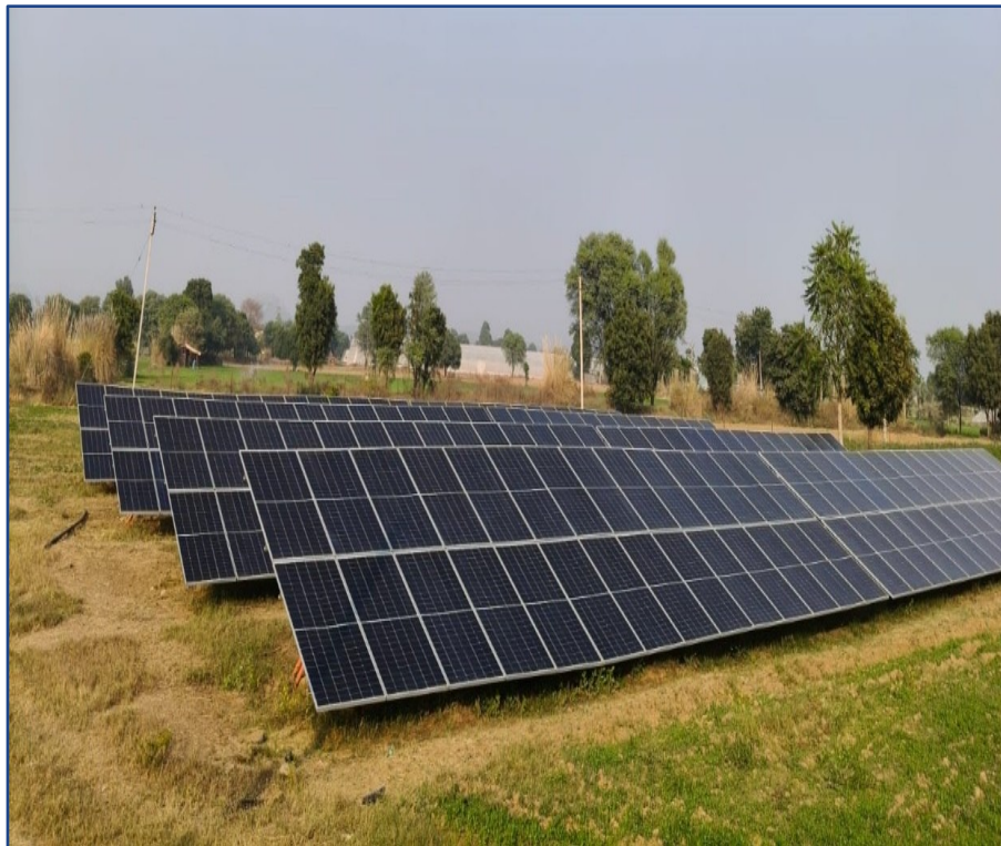
Figure 9: Ground Mounted Solar PV Plant in Kundanpura, Rajasthan
