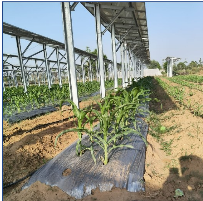
Figure 10: Retrofitted Elevated Agri-PV System (Energy +Agriculture) in Kundanpura, Rajasthan
