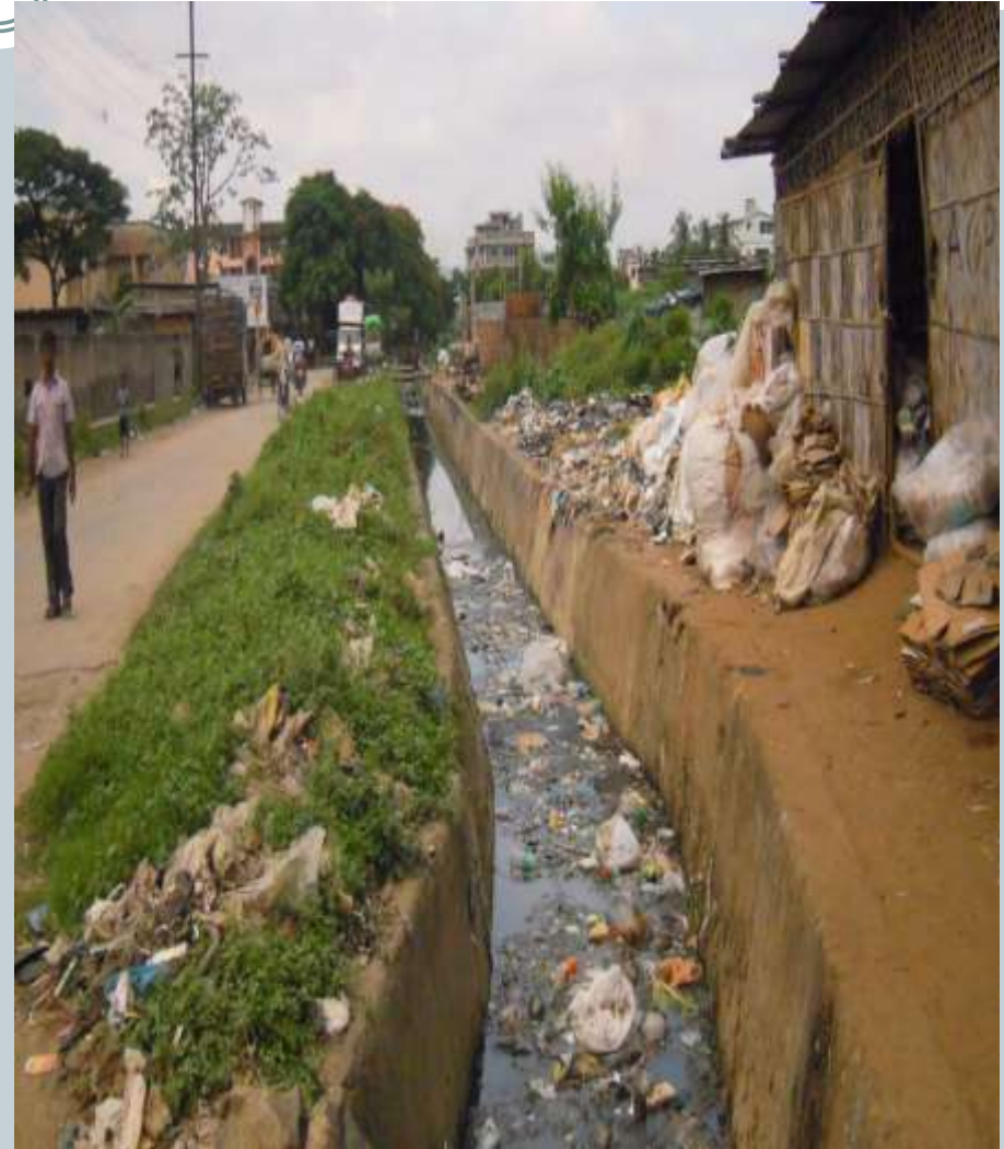
CLOGGING OF DRAINS
